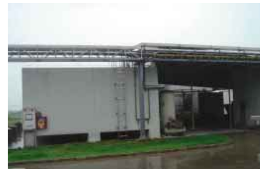
地上原水槽 Aboveground water tanks
