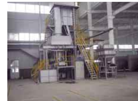
溶鉛炉 Lead melting furnace
