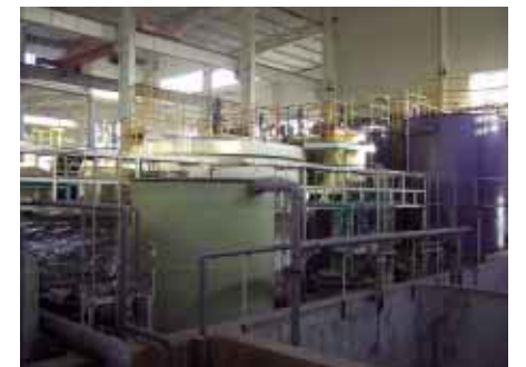
排水処理設備 Wastewater treatment equipment
