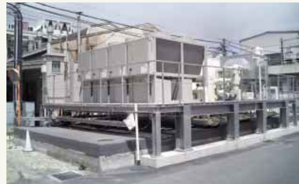
戻り水の冷却設備 Return water cooling facility
