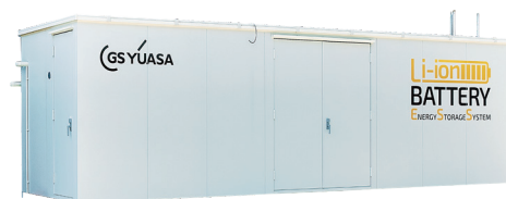
●Fig.1 Stationary Li-ion Storage Battery Installation
