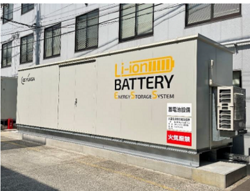
External appearance of the container type power storage system
