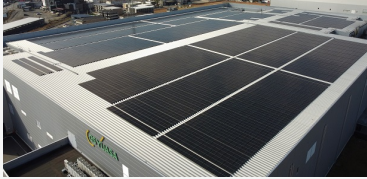
Solar power generation equipment (Ritto Plant)
