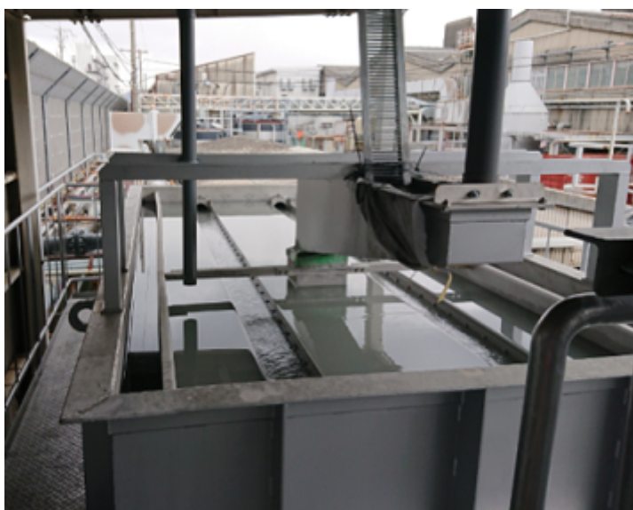
Installed high-speed sedimentation equipment
