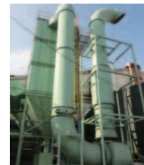
3 Upgraded dust collector 更新后的集尘机
