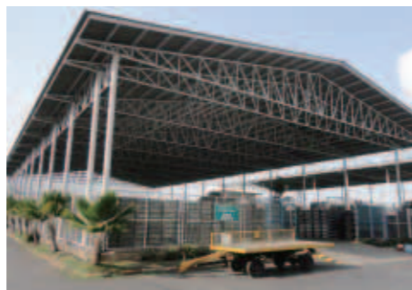
2 Roof over the lead alloy storage yard 铅合金保管场所的屋顶
