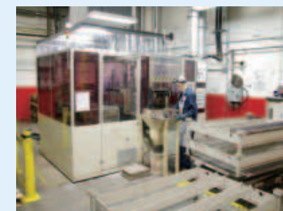
New battery plate parting system 新极板裁断装置
